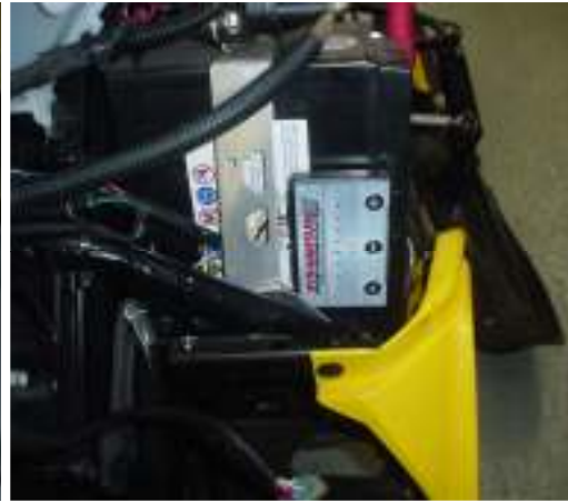
Programmer Mounted under Hood on Battery
